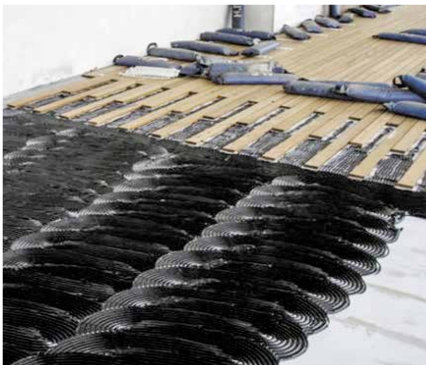
Fig. 40 A teak floor being laid, showing the bedding compound and the weights to hold it in place
