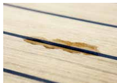
Fig. 58 Discolouration of the wood is a tell-tale sign of a failed or damaged joint in this teak deck
